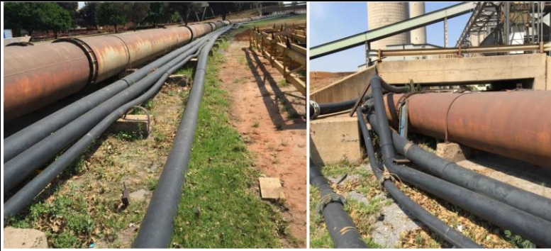
Figure 8: Current State of the Pipe Supports on Site
